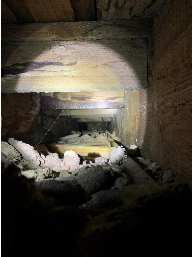
Figure 5 – Roof void below drip showing wet area at bottom of noggin and new timbers supporting a recent ceiling repair.
