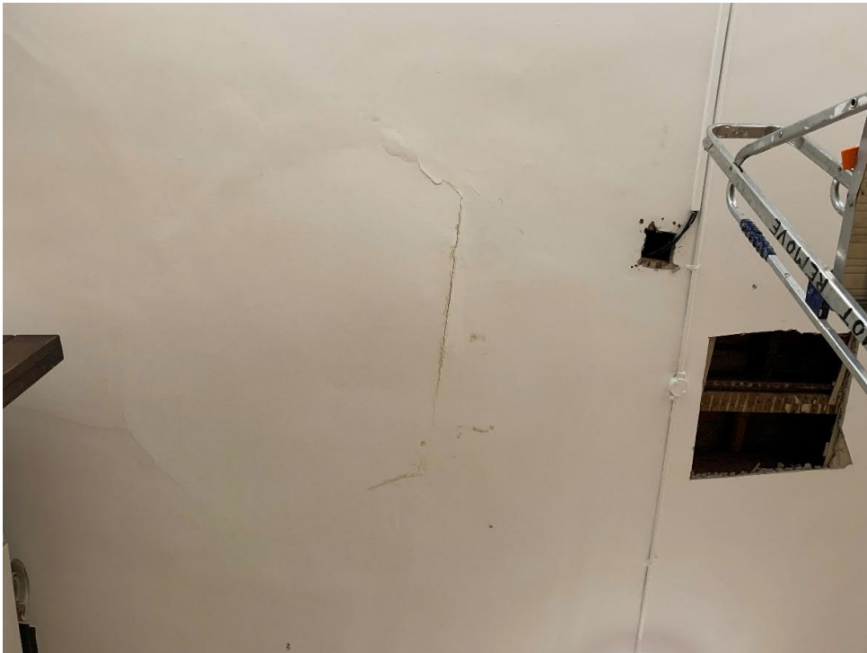
Figure 4 – Vestry Ceiling showing crack and bulge.
