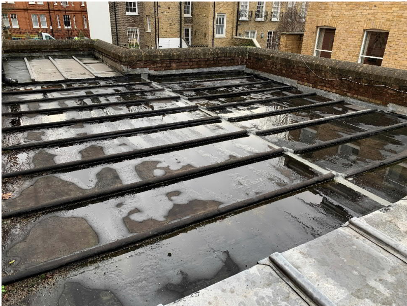
Figure 6 – Vestry Roof Covering. Central section covered in bitumen. The roof pitch is very shallow and there was a lot of standing water.
