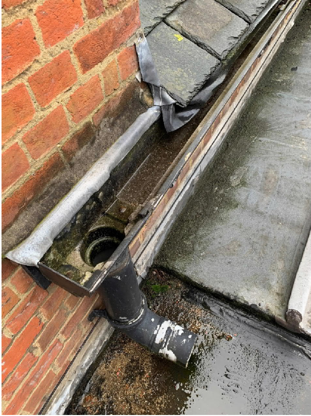
Figure 9 – North Aisle gutter discharging onto vestry roof.
