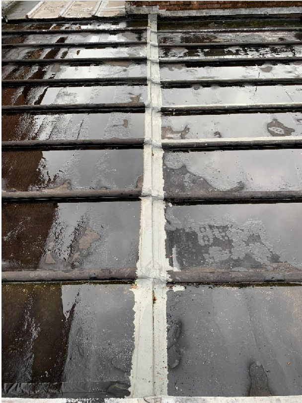
Figure 7 – Showing drip with Westwood PMMA waterproofing system applied in November 2023.
